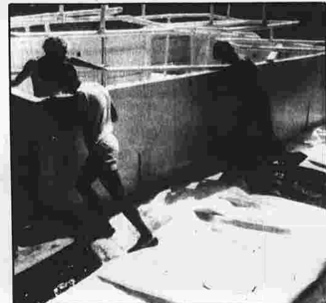
NEW METHOD — Bob Edwards of Andover, Peter Pouchel of Coventry and Chris Wilson of South Windsor install a "LayerAir" circulator this past summer at Lake Shennepit. The circulator, which can handle 40 million gallons of water per day, is used in a new process for redistributing oxygen in drinking and recreational water supplies.
